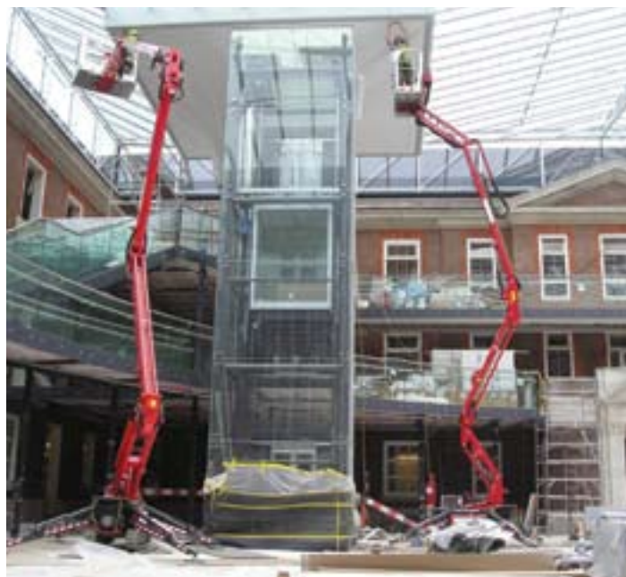
A 16 m RAM (left) and 14 m Hinowa machine owned by Tracked Access working on an extension to Middlesex University buildings at Hendon in London. Low floor loadings required the use of very large spreader plates.
