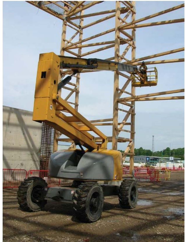
Figure 1 Operating a MEWP near overhead structures
