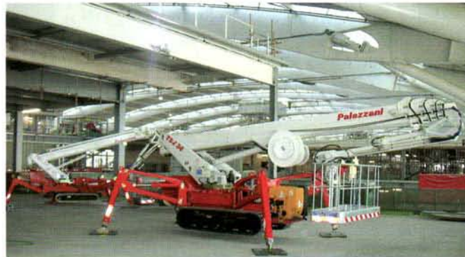
Tracked Access Ltd has supplied two of its Palazzani tracked platforms to assist with the fit-out of the new Terminal 5 at Heathrow Airport.
